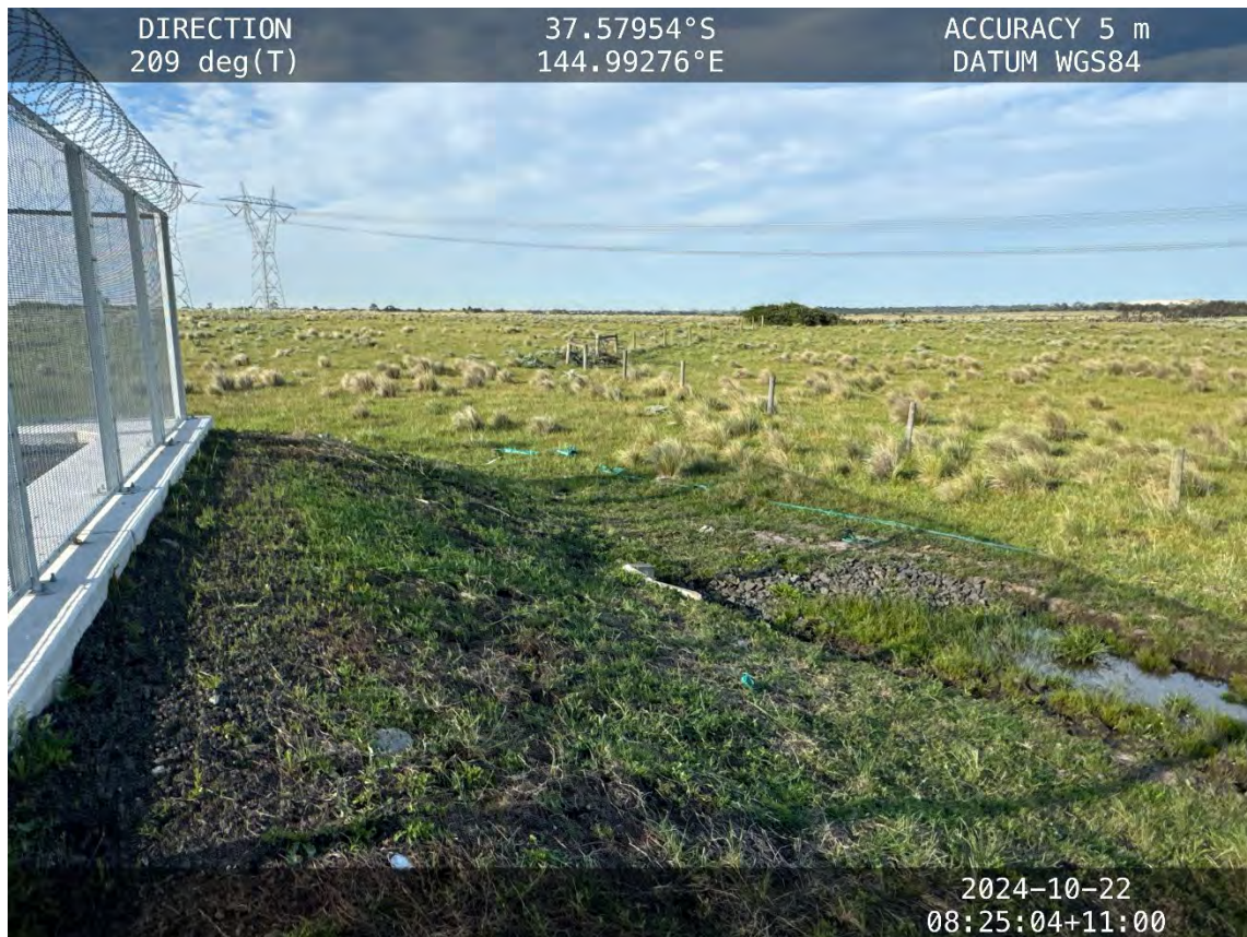
KP50 Wollert Compressor Station - base of batters around new compressor area with damaged and strewn sediment fencing.
